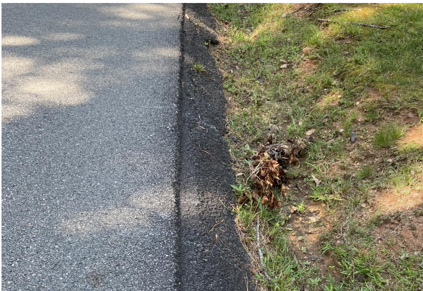
Photograph 7: Sloped pavement edge near Young Manor Drive
